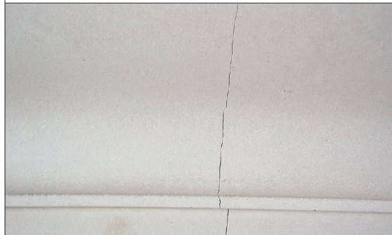
A Surround without Fiber Reinforcement Exhibits Cracking During Thermal Testing
